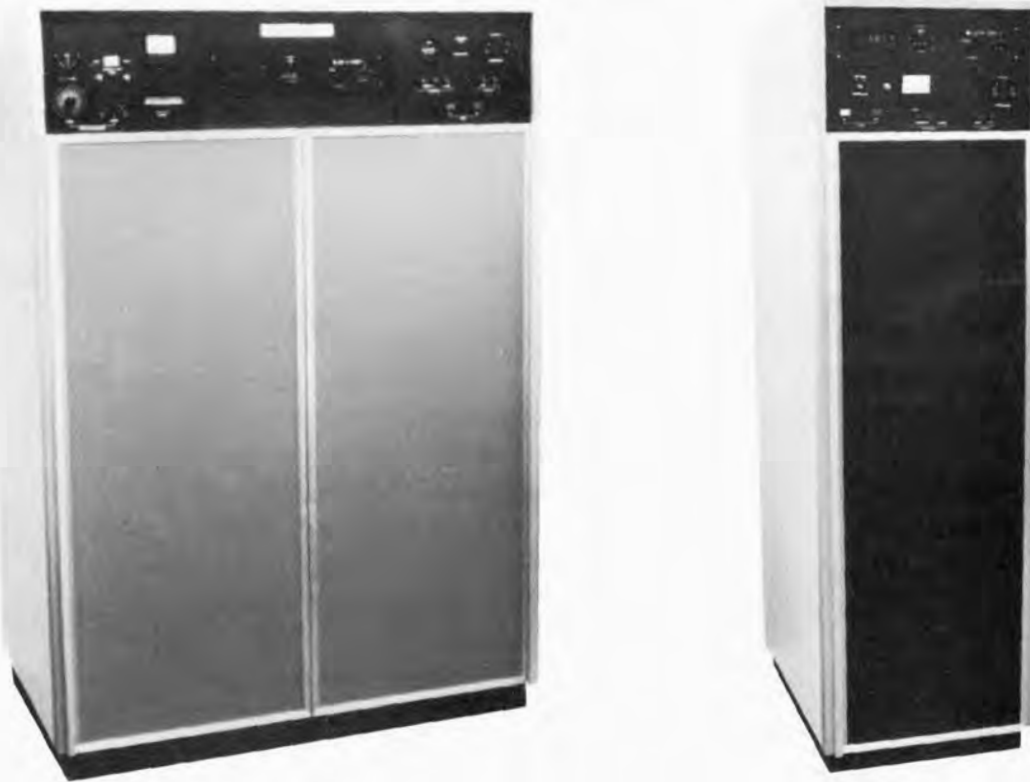
Figure 1-9. Power distribution units
